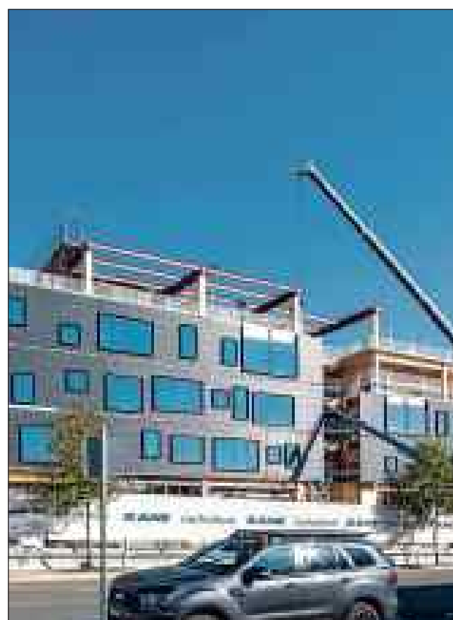
NEW WORKPLACE: The Govhub building will house up to 1000 Victorian Government employees, including up to 600 public sector positions relocated from Melbourne. Picture: Luke Jarvis, John Wardle Architects.
